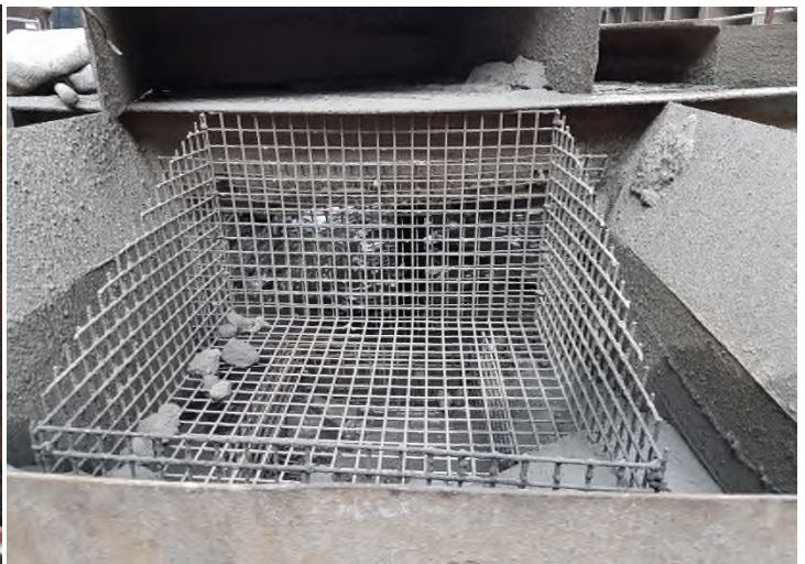
Figure.2 – mesh baskets fitted to receiving tanks
